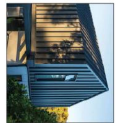
MATT COLORBOND STANDING SEAM METAL CLADDING
